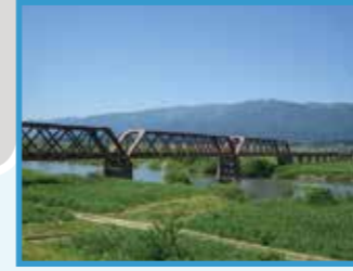
The Arato Railway Bridge, still functional after a century, with the Mogami River flowing by
